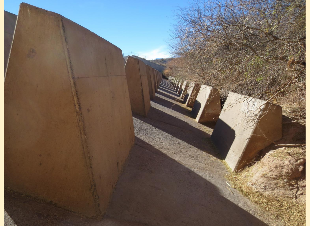
Figure 5. Picture of baffle blocks located in the San Simon Barrier Dam outlet structure.
